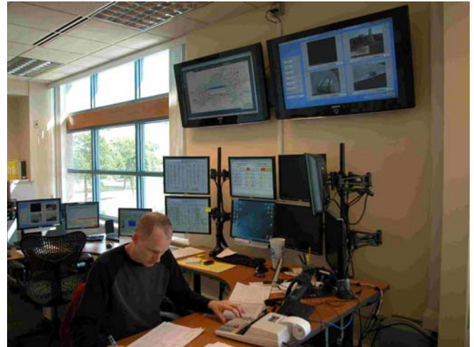
Figure 1: Video from 32 remote sites is sent via wireless to the central control room at the Madison Water Utility in Madison, Wisconsin. The video uses the same wireless link as the SCADA and access control system, and the video images appear on a Wonderware HMI system.
